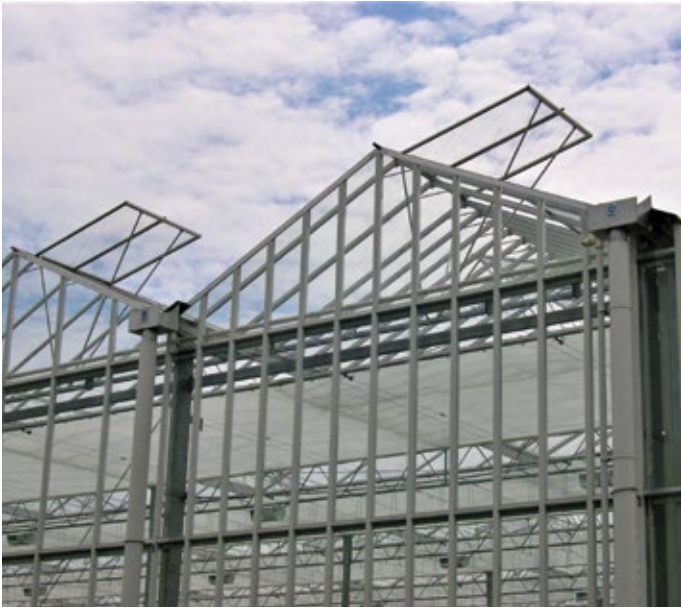
Roof vents wide open on a hot day
