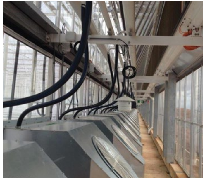
Corridor from Enerdes
